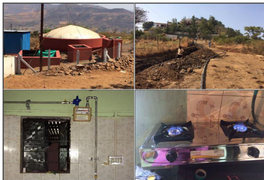
Biogas Cooking Grid at Gawaliwada, Pune
