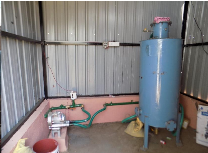
Scrubber in control room
