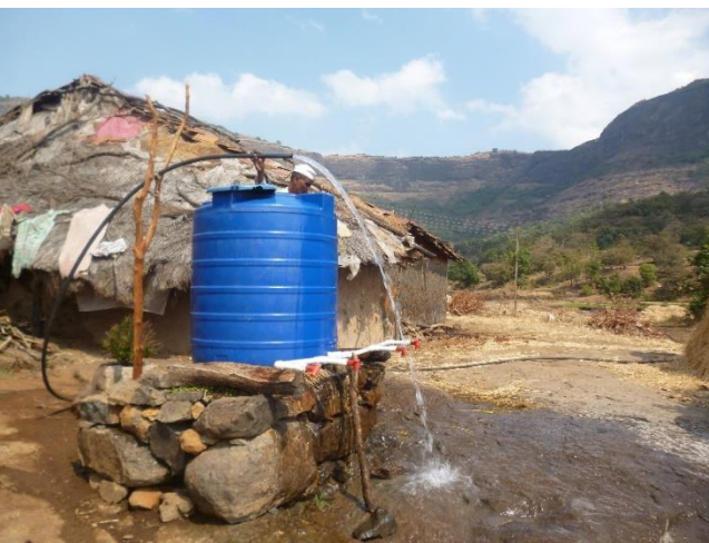
Water Pump, working on microgrid
